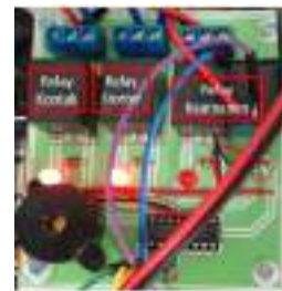
Gambar 10. Uji Coba Relay Starter
